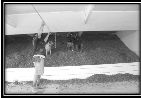
Volunteer workers Craig Jenkins, Mike Jackson, Jeff Taylor and mascot laying Sheetrock (range).
